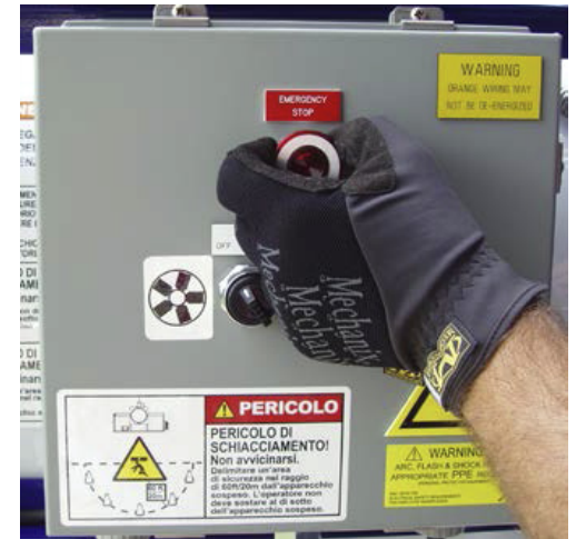
Emergency Stop - Control
